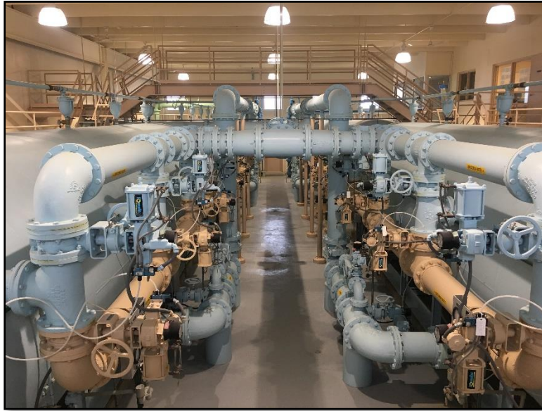
Water Treatment Facility – Interior
