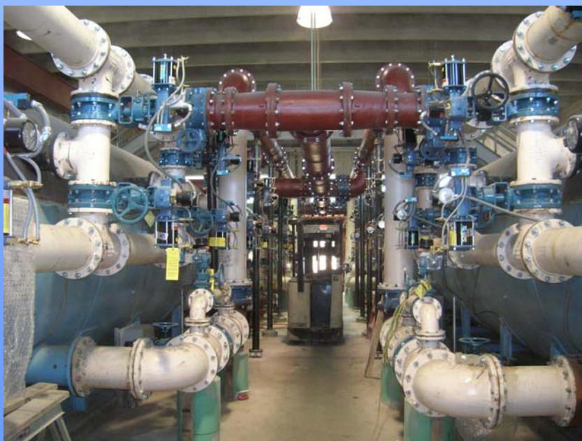
Water Treatment Process Piping, Delano Water Treatment Facility
